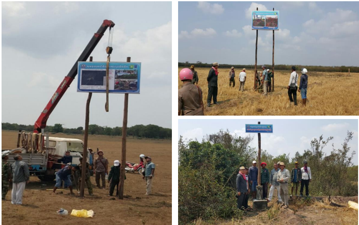
Figure 3: Boundary concrete poles attached with banners and billboards installation at replanted area
